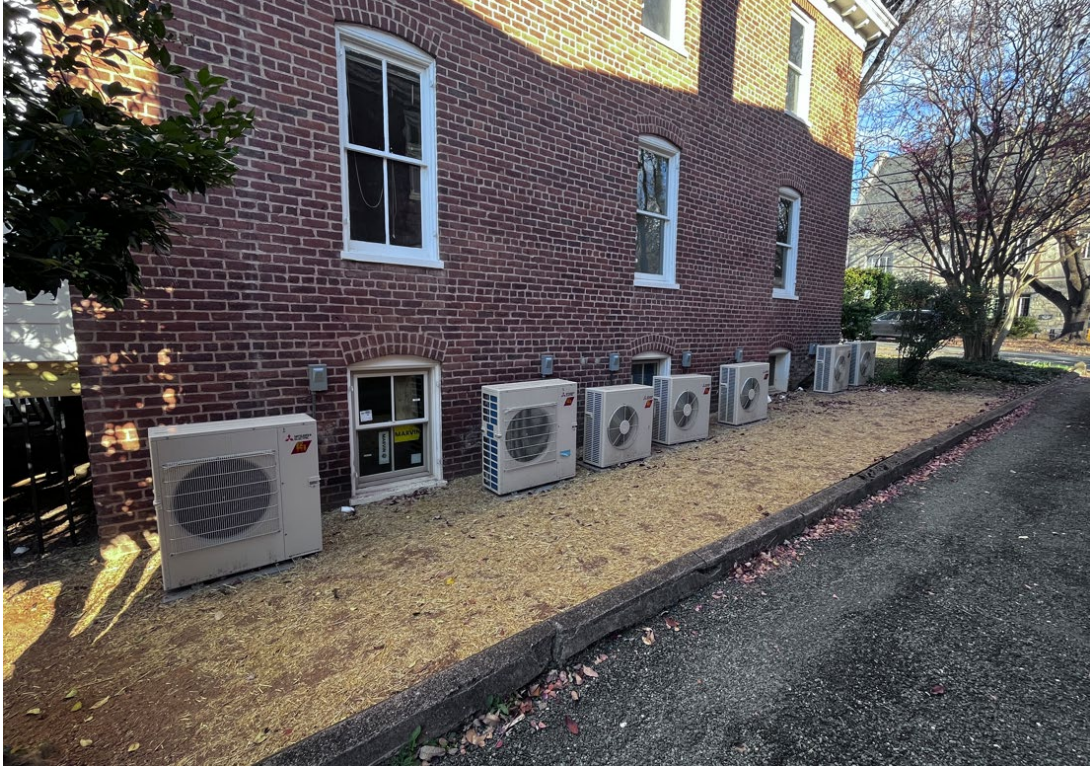
Mechanical units at side yard, November 2024
